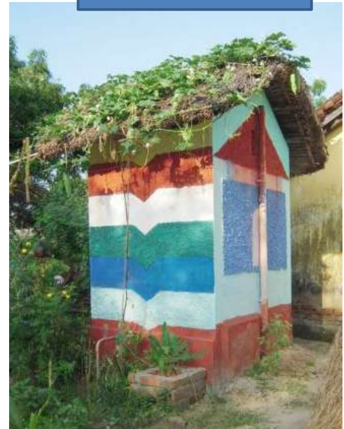
Innovative roof but faulty vent pipe
