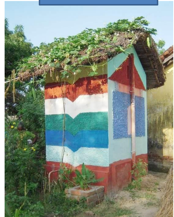
Innovative roof but faulty vent pipe
