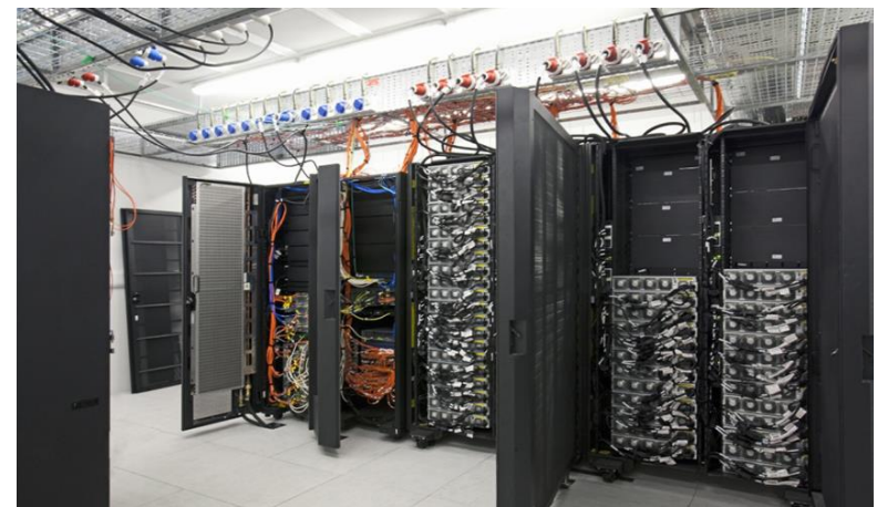
The CY-TERA HPC facility
