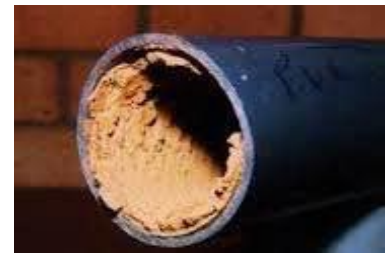
Fig.27: Incrustations in a water pipe
