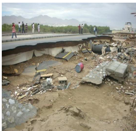
Figure 8: Street damage in the aftermath of cyclone Gonu in Oman, 2007
