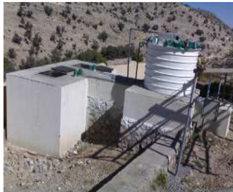
The constructed treatment system in Al Jabal Al Akhdar, Oman
