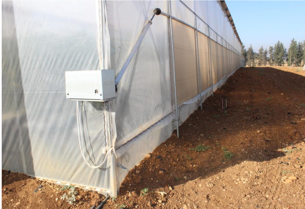
Automatic Ventilation System
