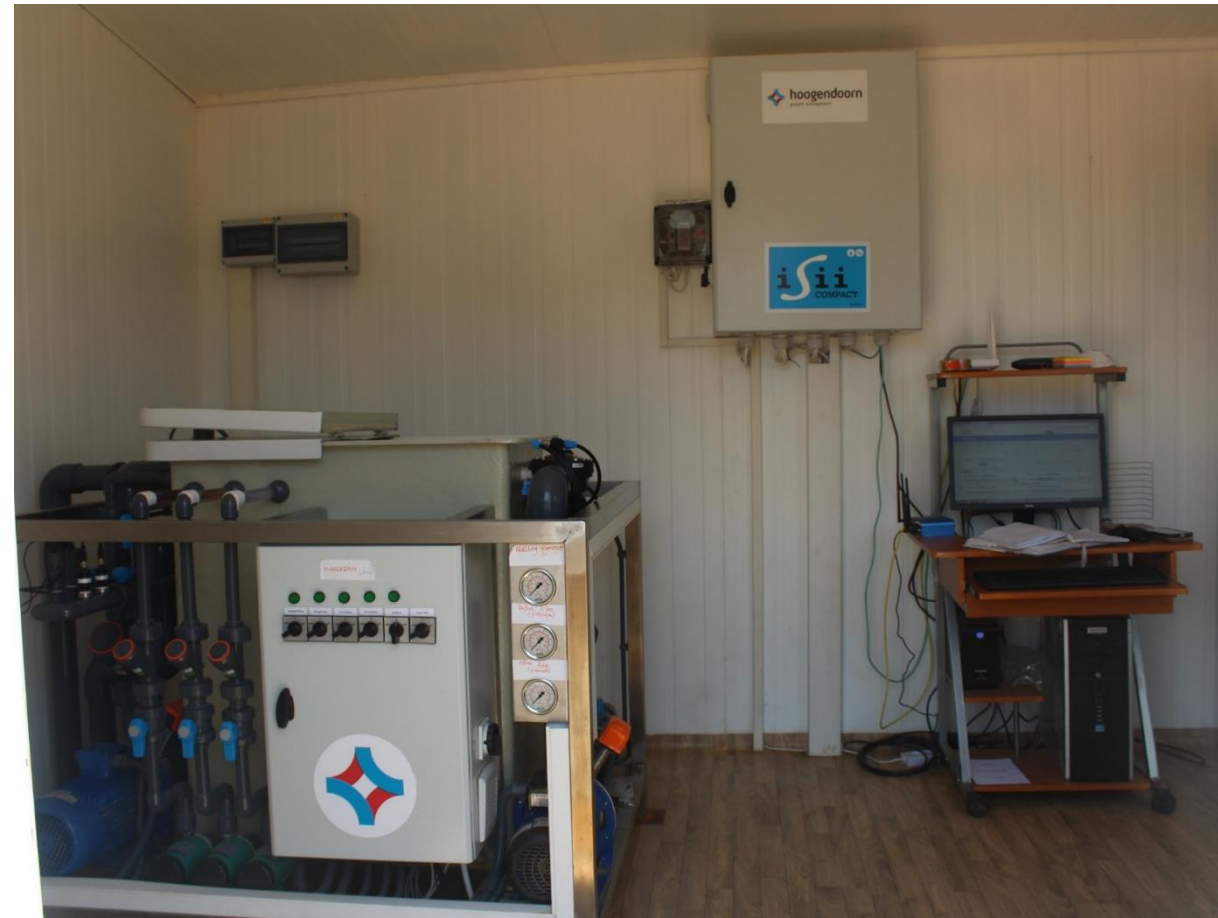
Automated Fertigation System
