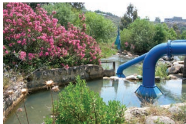
The Wazzani pumping station, Lebanon, 2006. Source: Eileen Maternowski.
