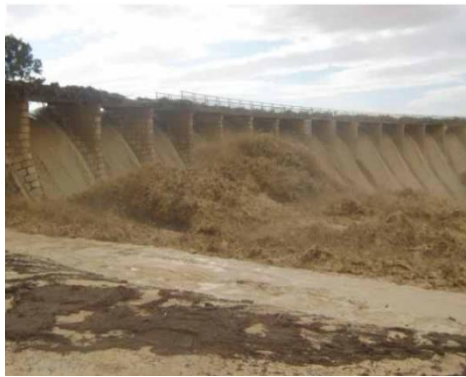
Fig. 1. Al-Rwafaa Dam in Jan. 2010 Flash flood
