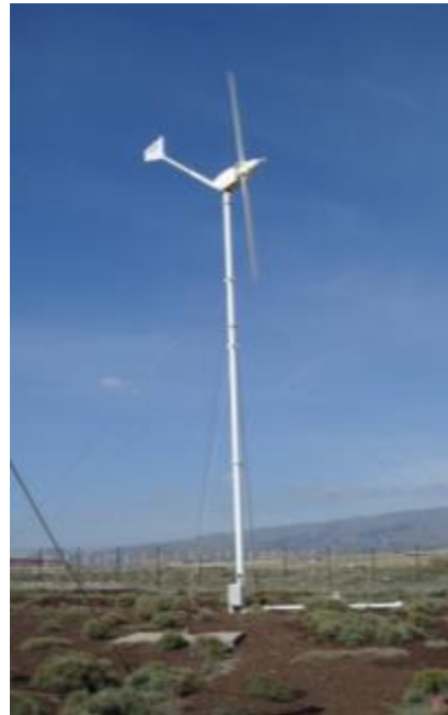
Wind turbine (15kW).
