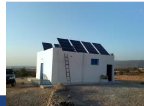
PV field (4 kWp).
