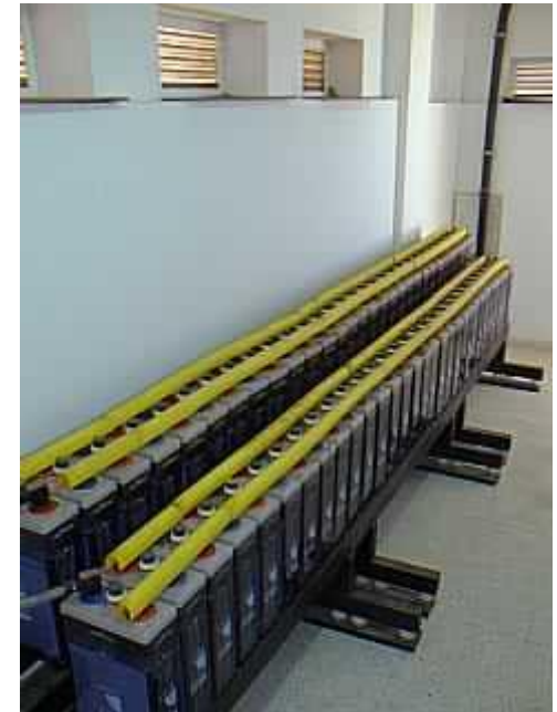
Battery bank (23 kWh).
