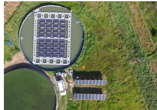
Solar panels in WWTP Lianyungang, China
