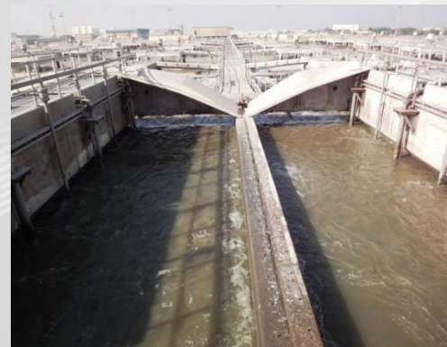
Grit Removal Tank
