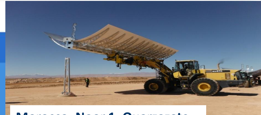
Morocco_Noor 1_Ouarzazate 160 MW in operation Jan 2016
