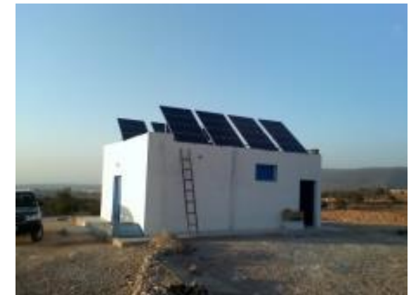
PV field (4 kWp).
