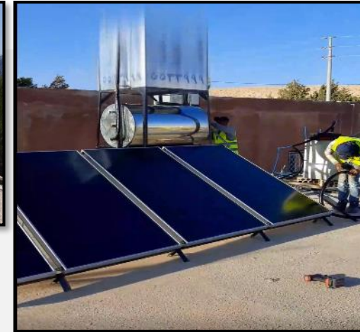
Solar water heating system in Maan
