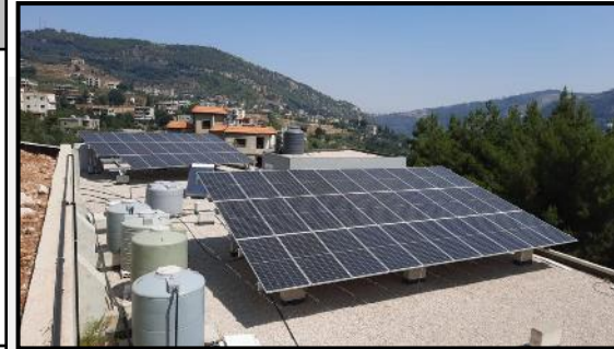
25 kWp solar PV system and solar water heating system in Akkar, Lebanon
