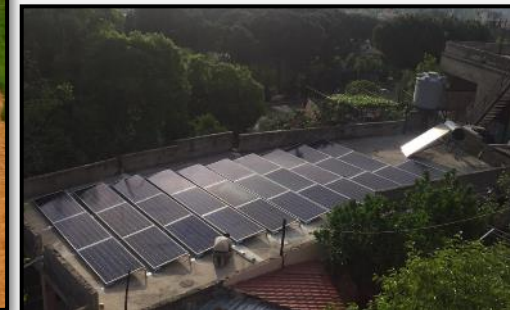
10 kWp solar PV system in Akkar, Lebanon
