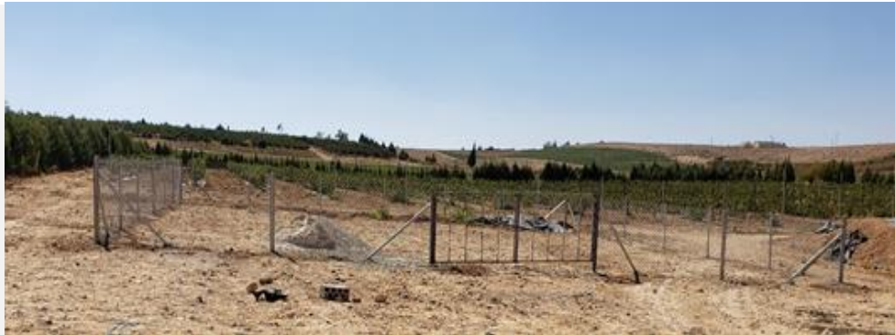
Project #1 (22 kWp): Solar PV on-grid ground-mounted system for the farm of Mr. Saleh Afash in Al- Achaari.
